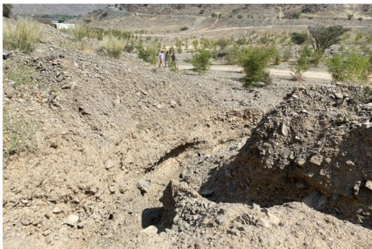
Fig. (7). A break in the existing contour ditch in ATF site, created by the last rainfall.
